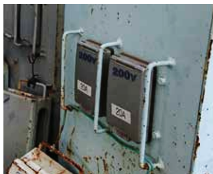
Shipbuilding (distribution board)
